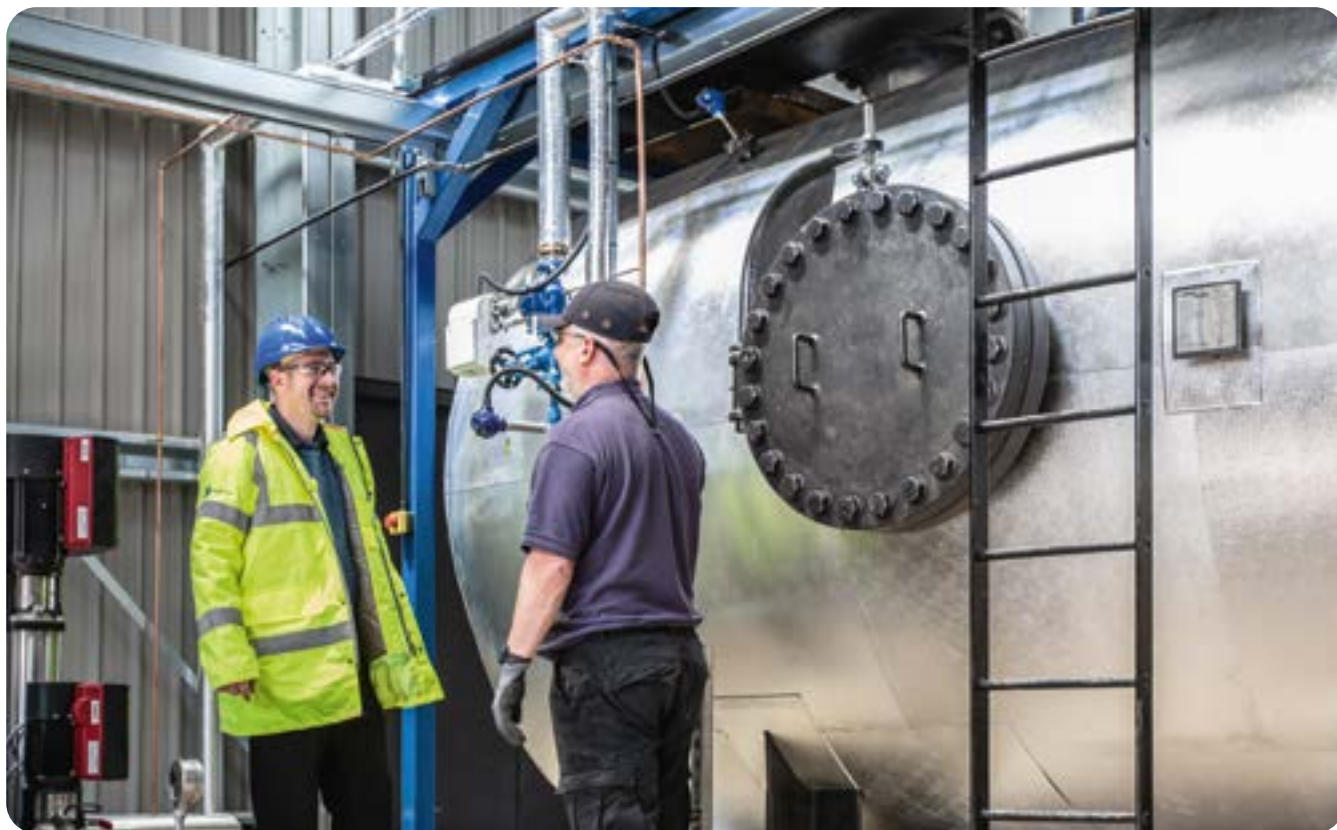
Steam Battery is part of our TargetZero decarbonisation solutions.
